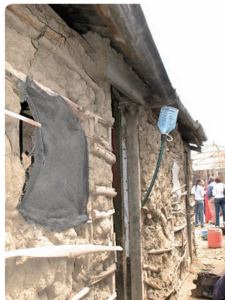
Improvised household rainwater harvesting system in Mirer-Karagita settlement
